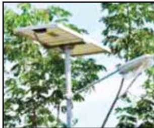
Solar panels power street light in L & T Campuses
